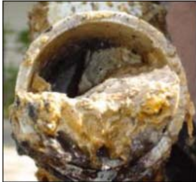
Figure 1. Sewer line clogged by restaurant grease: improper FOG management increases operation and maintenance costs for sewerage utilities.
