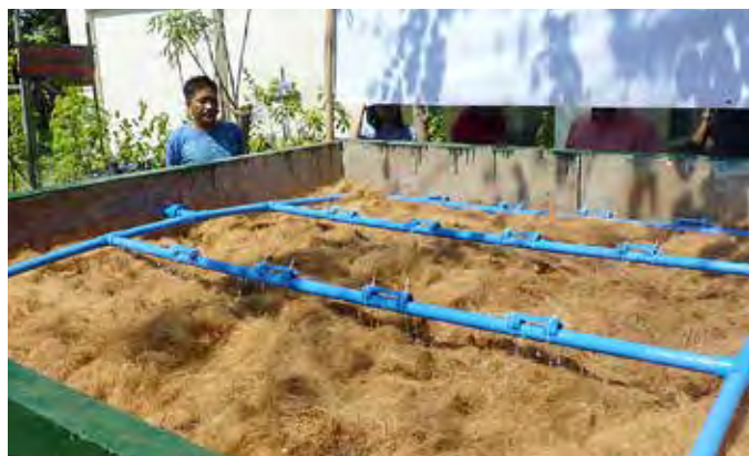
Cocopeat wastewater system installed for Putatan Elementary School, Philippines. The system serves 700 students for less than 1 US penny per student per day.
