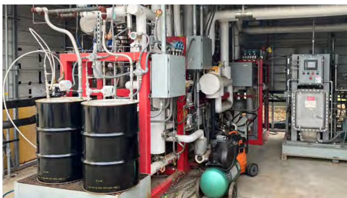
Gas-to-liquids process unit
