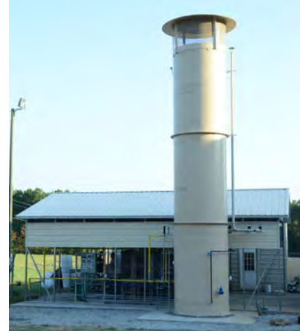
Enclosed flare stack
