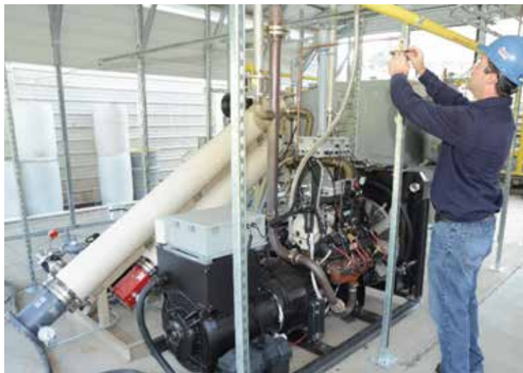
Current pilot of RTI Microreformer located in Research Triangle Park, NC.
