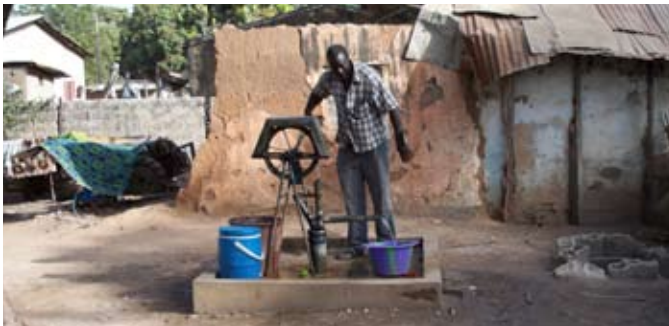
A hand-operated rope pump installation. This type of low-cost, hand-drilled well is an effective alternative to conventional drilling in some locations in Senegal. [Photo: Fathi Kraiem]
