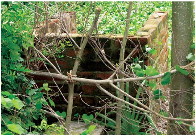
This toilet in Orissa shows that latrine structures can be simple and still offer privacy. [Photo: Katherine L. Dickinson]
